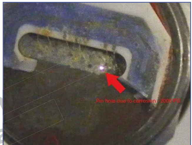
The pitting of a 316L pressure-sensor diaphragm 0.030 inches thick with less than one-month service near the Great Barrier Reef in Australia.
